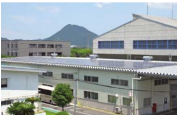
Photovoltaic power generation
