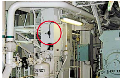
Beside generator engine
