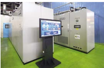
Power recovery system
