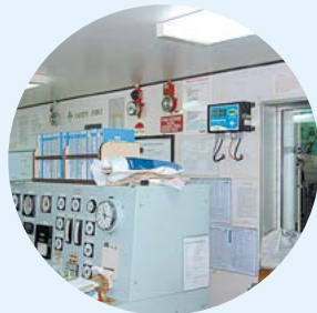
Engine control room
